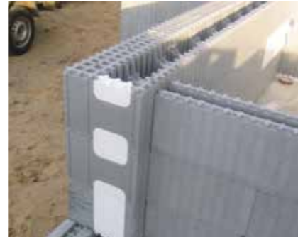
While constructing reveals and blunt wall endings, close up openings in the formwork with OH, OB and OC elements.
