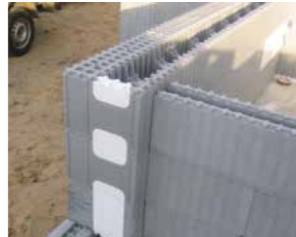
While constructing reveals and blunt wall endings, close up openings in the formwork with OH, OB and OC elements.
